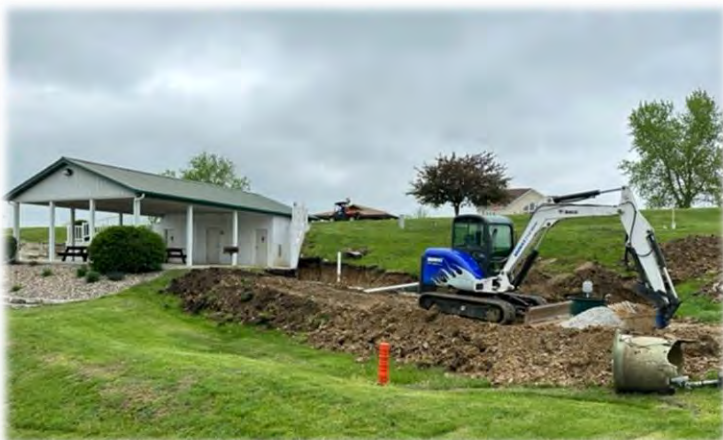
Work was done to remedy the drainage situation at the Beach House.
